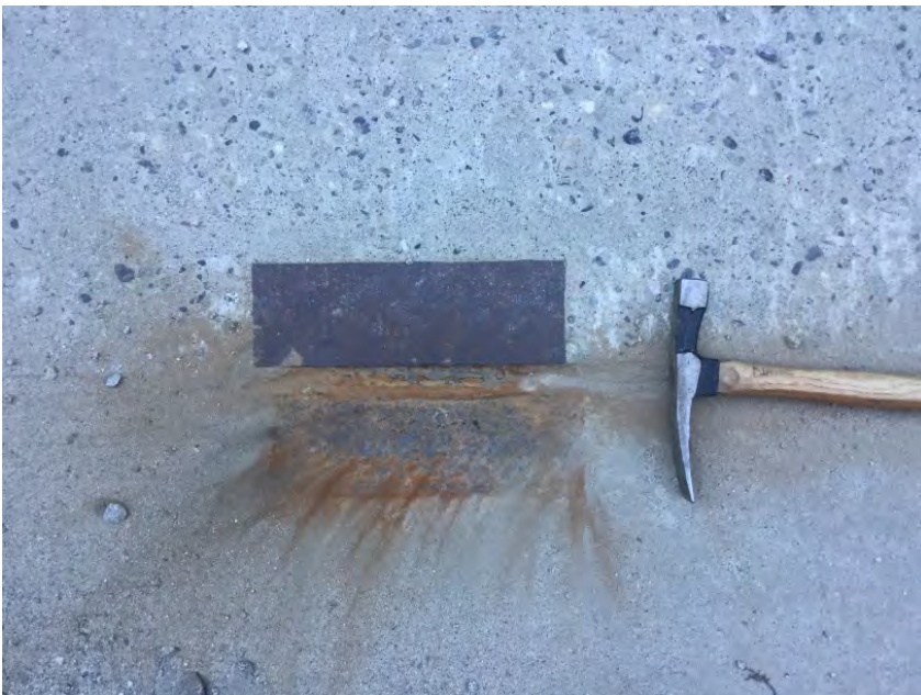
Minor Misalignment of Shear Connector
