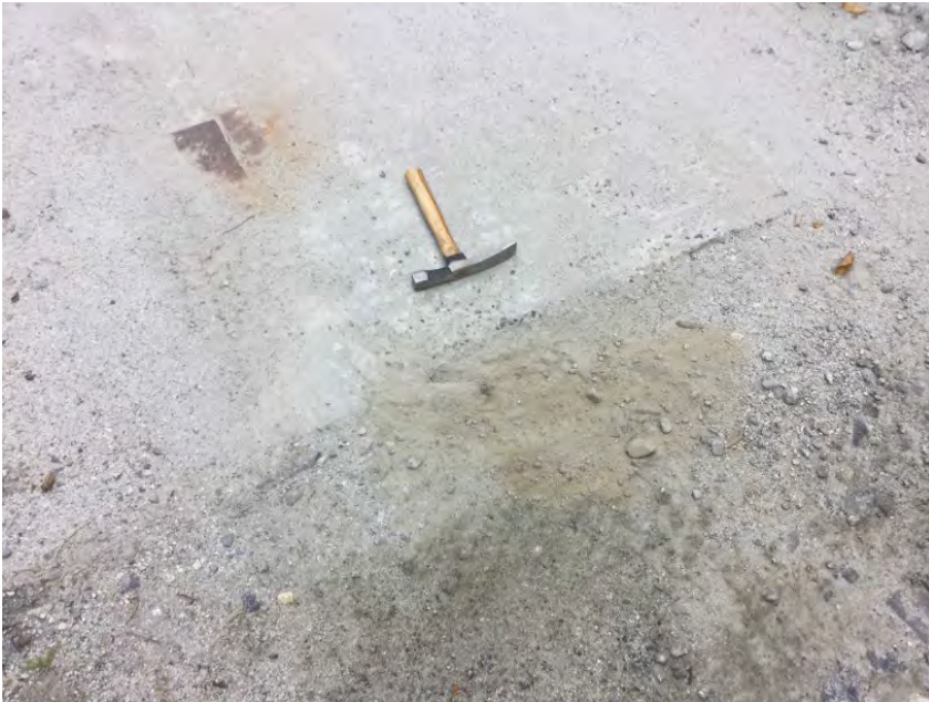
Minor Damage to End of Slab at Approach
